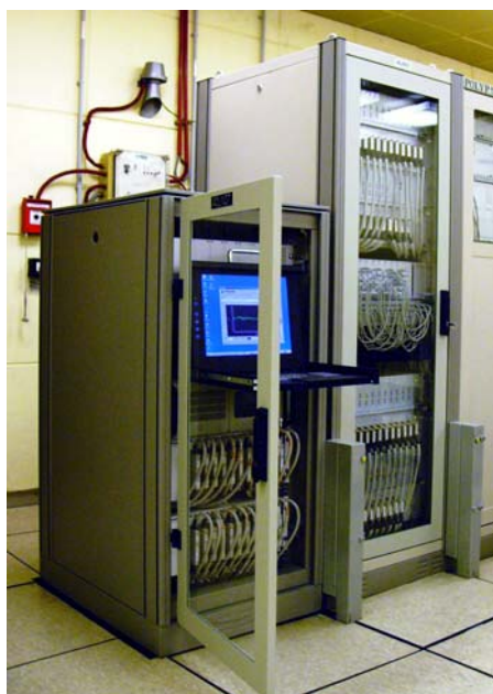
Fig. 1. Implementation at Unit 4. Computer and multiplexers are in the smaller rack, while signal conditioning modules are in the larger one
